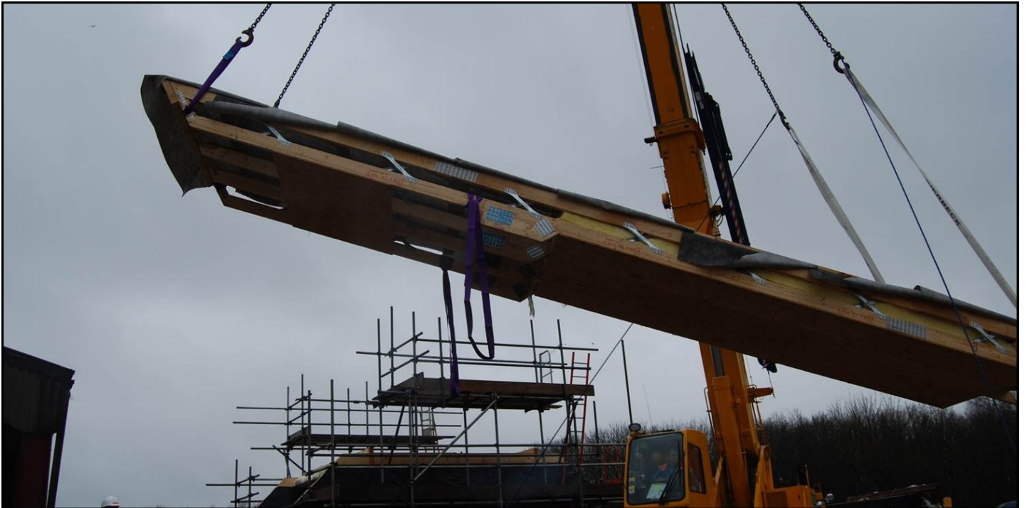
Pre-Insulated, felted and counter battened offsite, the X-Rafter cassettes are craned into position.
