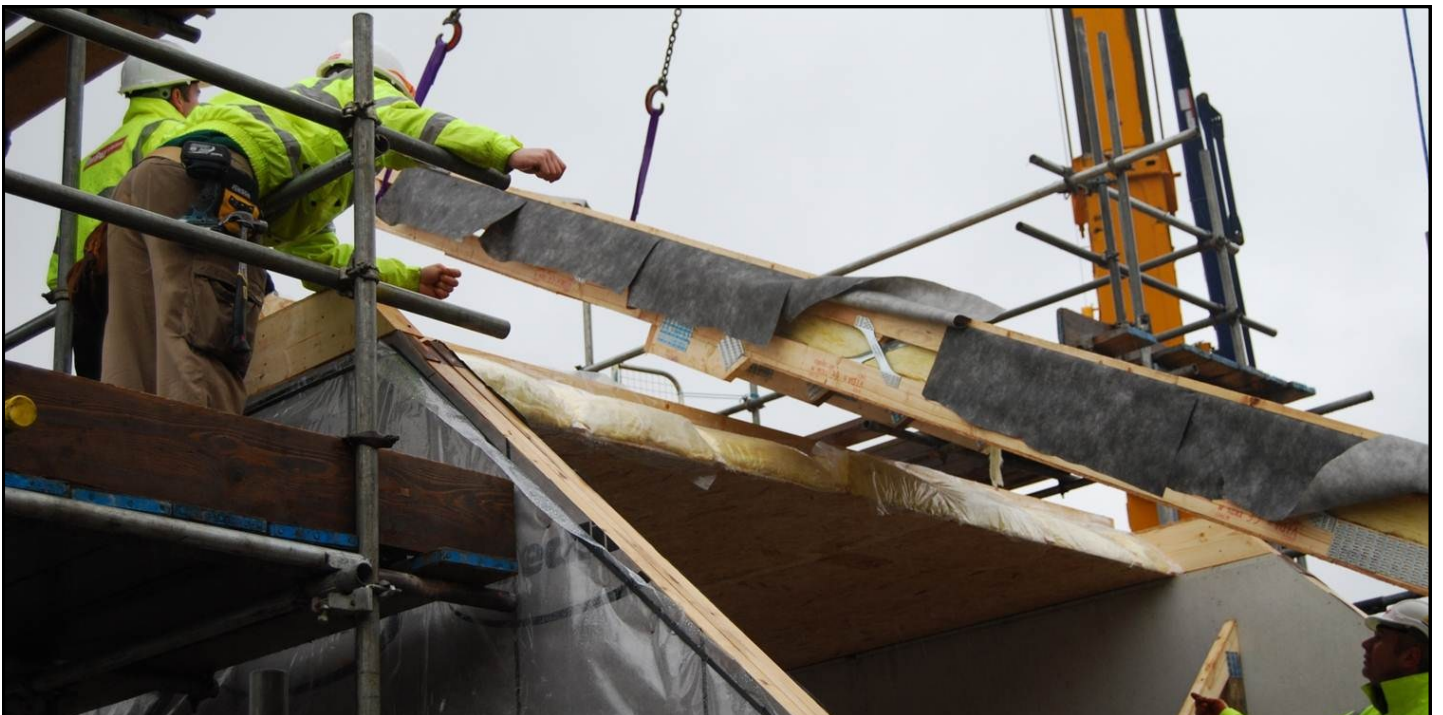
The Posi-Joist cassette floor and the structural ceiling cassettes form two safe working platforms providing that the appropriate harnessing is worn by the installation team.
